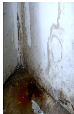
Mold damage caused by water intrusion
